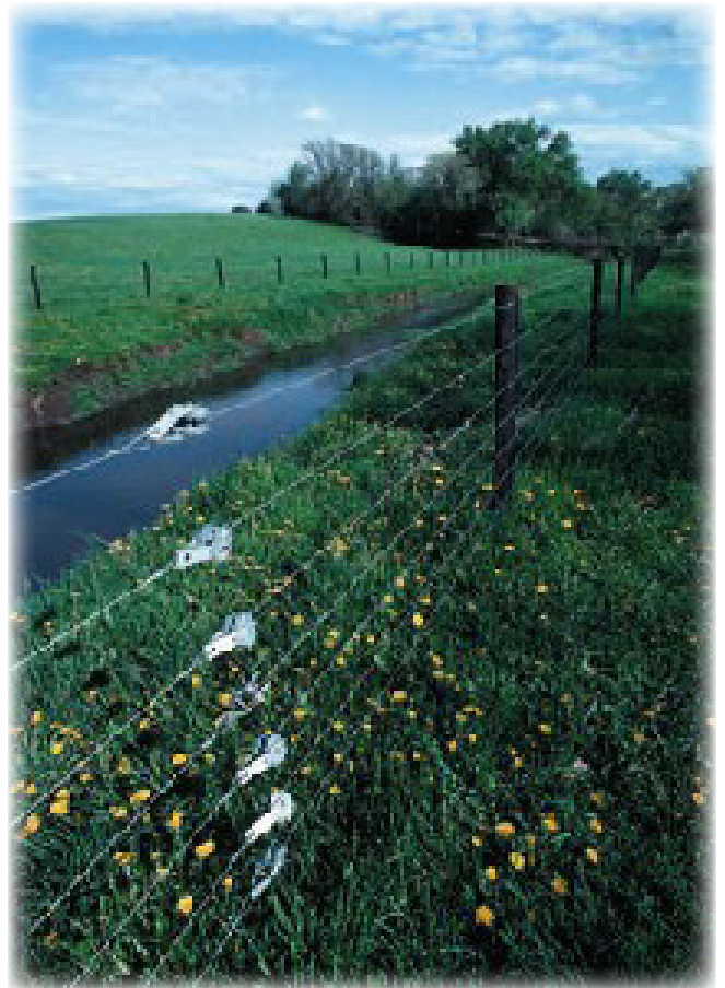
Permanent fence installed to create vegetated stream buffer. Photo courtesy of USDA NRCS.
