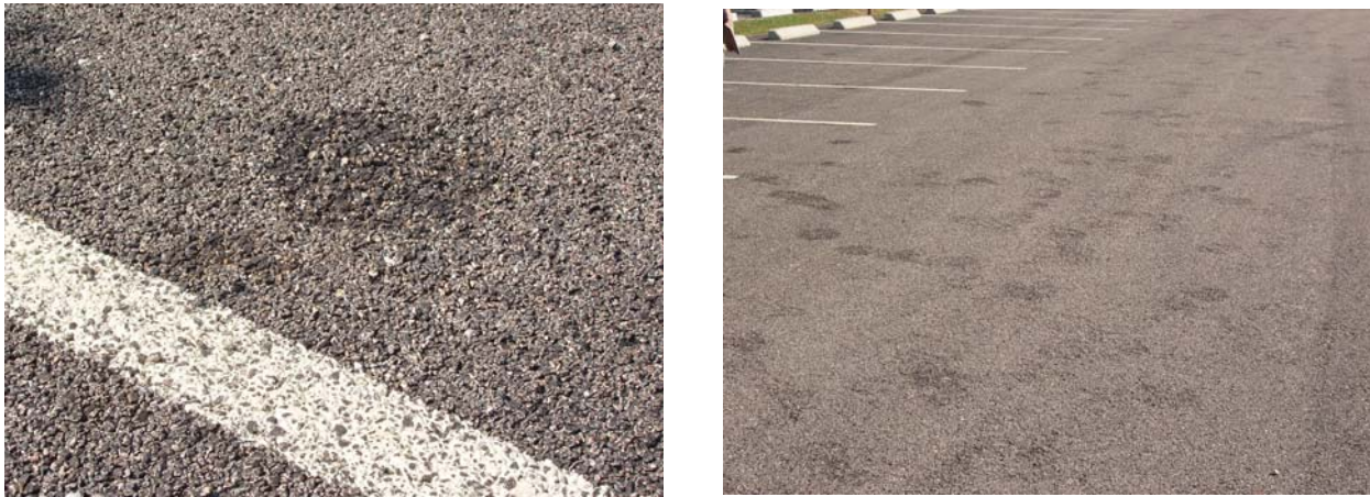
Figure 7. Surface defects have appeared within the parking lots. The left photo shows a close-up view, while the right photo shows a particularly damaged area.
