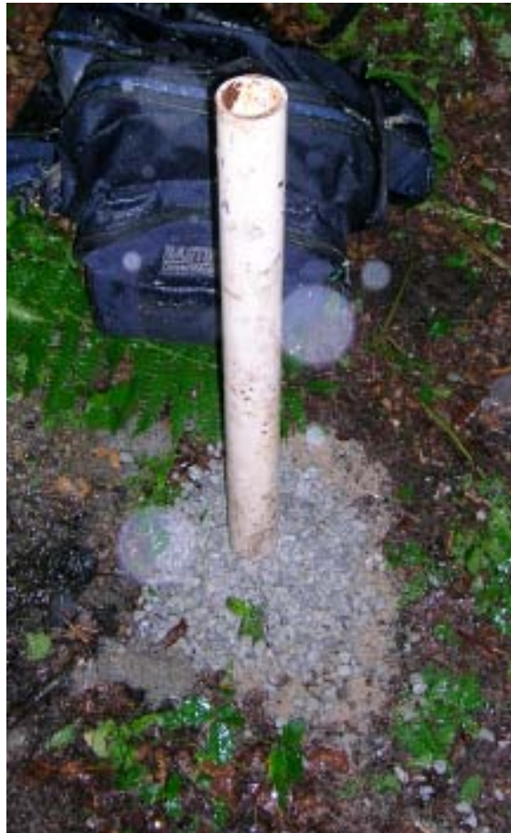
Figure C3: The installed well. The blue pellets surrounding the well are the bentonite
