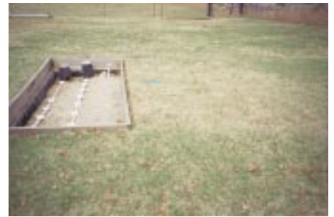
Part of this single pass sand filter is exposed at URI's On-Site Wastewater Training Center for demonstration purposes. It is one example of an enhanced treatment component approved for use in Rhode Island.
