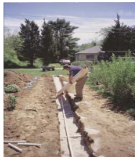
The shallow, narrow drainfield design is a typical component of the enhanced treatment system.
