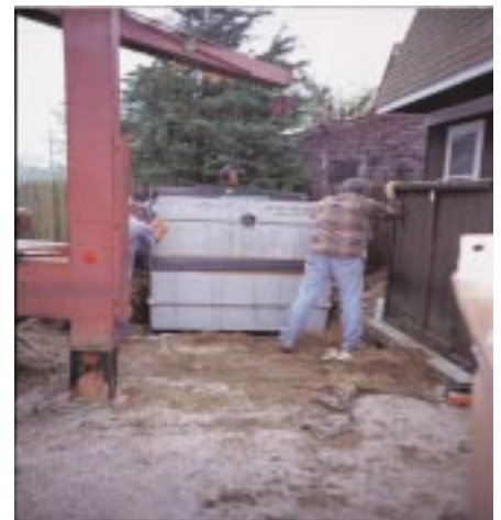
The seam of this concrete septic tank is sealed with a butyl strip that provides additional assurance that it is watertight. The inlet and outlet have cast in place rubber boots with stainless steel clamps.
