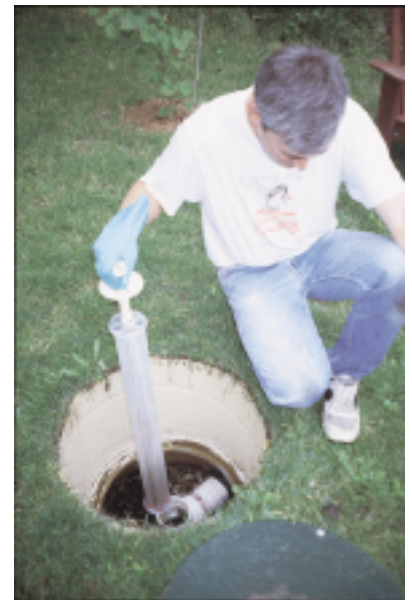
Access risers installed to grade allow for ease of maintenance and inspection. Here the effluent filter is being reinstalled after being cleaned.
