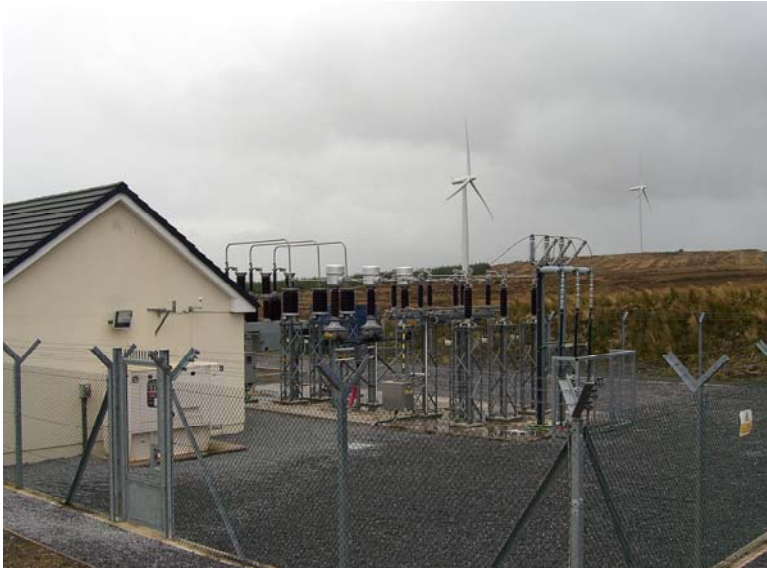
Transformers at the Taurbeg Wind Farm, Ireland
