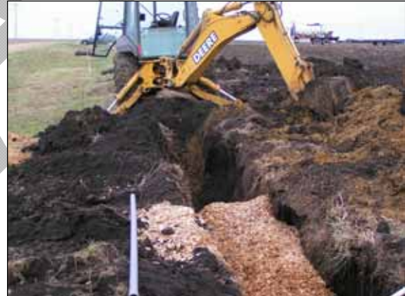
Placement of woodchips into a trench to prepare a bioreactor system – Univ. of MN
