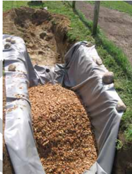
Water infiltrating into the first retrofitted area with the drainage pipe will flow into a woodchip bioreactor. The bioreactor consists of an impermeable geotextile liner filled with woodchips. Its function is to denitrify the infiltrating water.
