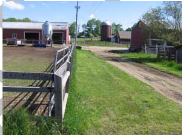
The grassy area between the fence and road was utilized for placement of the woodchip filled bioreactor.
