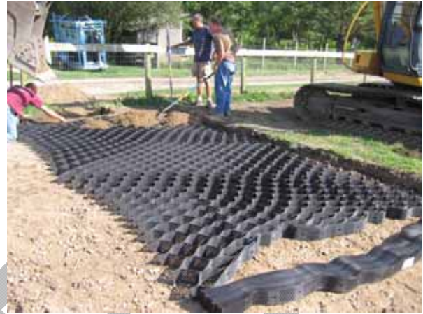
Process gravel is placed over the geotextile, the geogrid system is then placed and backfilled with additional process gravel.
