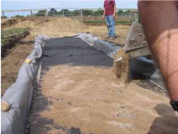
First test area is excavated and an impermeable liner is placed along the native soils. A drainage pipe is then placed along the middle of this cut to collect water infiltrating through the system. Crushed stone is placed over and around the drainage pipe over which geotextile is placed. Chip sand is placed over this geotextile (see image) and separated from the overlying geogrid system by another layer of geotextile.
