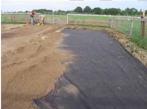
The second test area is retrofitted by placement of geotextile over the native soils and then backfilling with process gravel.
