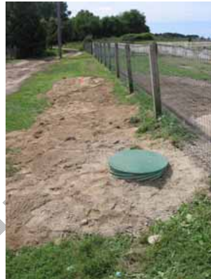
The bioreactor influent can be sampled from the distribution box which is accessed from the manhole.
